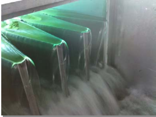
UV Disinfection Effluent at WWTP
